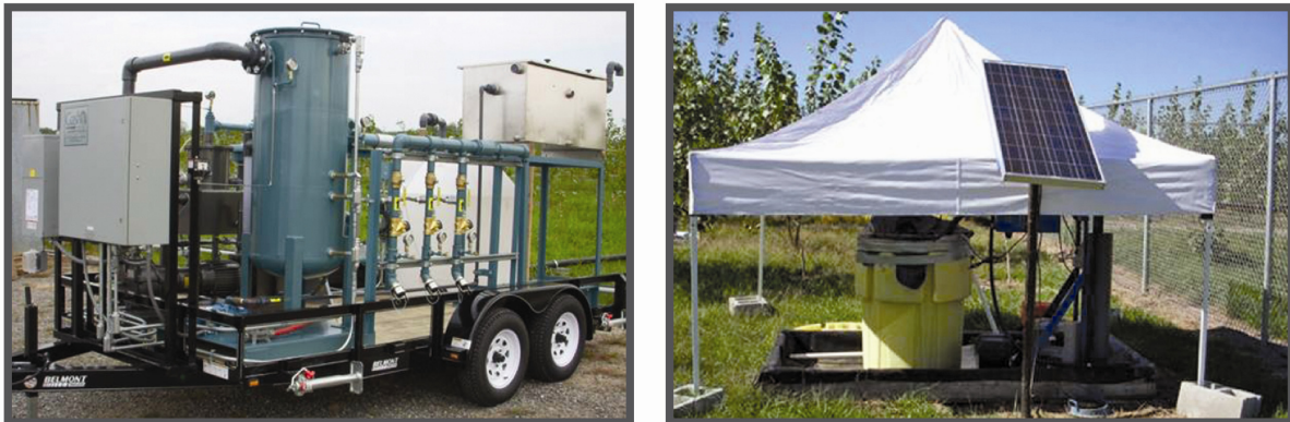
Figure 7.6. Examples of site remediation systems showing a multi-phase extraction unit (left) and a solar-powered belt skimmer at a Superfund site in the eastern USA (Photographs courtesy of B. Butler, ERM).
